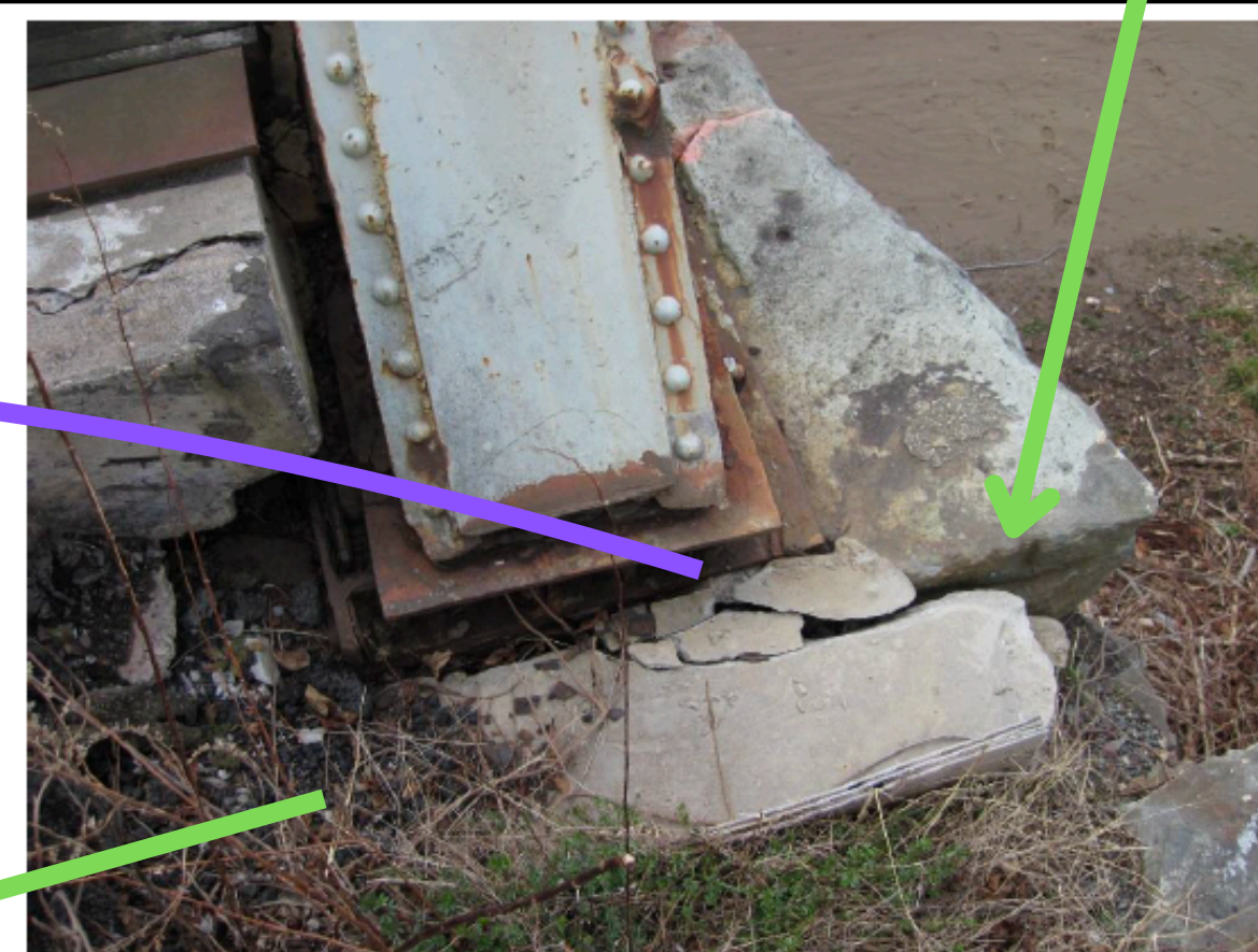
8. Far left truss bearing, looking back. Note cracks in the (2018) concrete repair.
