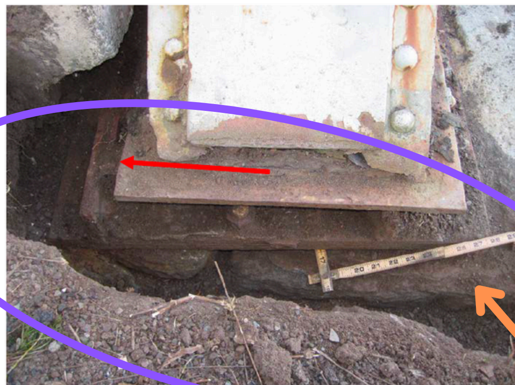
54. Detail of previous photo. Note the truss is shifted laterally to the left and the cap stone is fractured and settled underneath the bearing.
