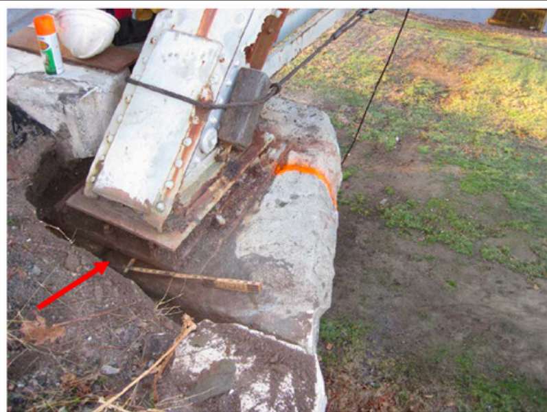
53. Left truss expansion bearing at the far abutment, looking back. Note the rollers are frozen and the truss is shifted laterally to the left. Also note the lateral probe below the masonry plate and fractured cap stone.
