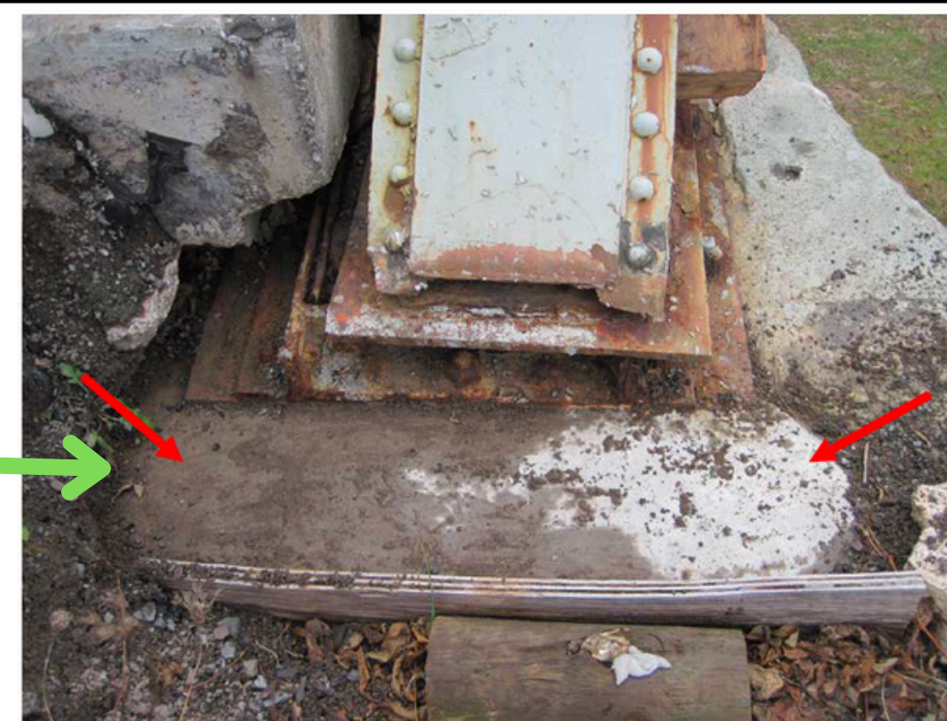
55. Left truss bearing at the far abutment, looking back. Note the grouted repair on top of the fractured cap stone (work done).
