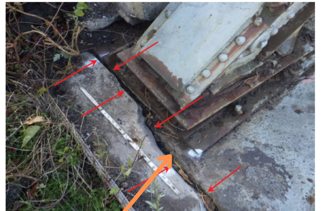
80. Repair done in 2018 adjacent to the Left Truss bearing showing evidence of movement
