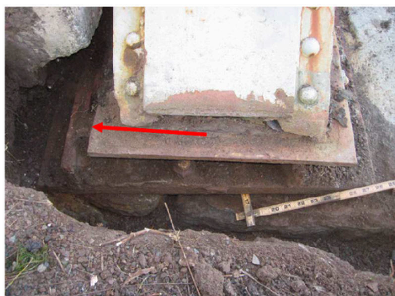
54. Detail of previous photo. Note the truss is shifted laterally to the left and the cap stone is fractured and settled underneath the bearing.
